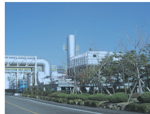
Exhaust Air Purifying System (VOC/Odor Treating System)
